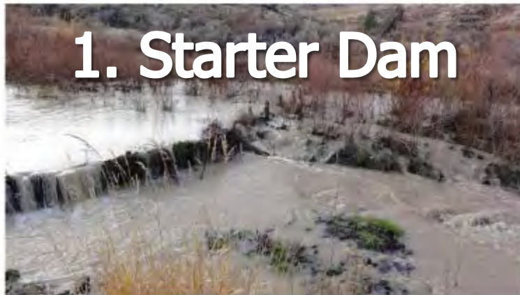
Figure 10. A typical starter dam (SF-17 at sunflower) with willow branches woven between vertical posts and the back side sealed with rock and clay. Note the dam height is sufficient to divert flow onto the RL terrace, mimicking a stable beaver dam.
