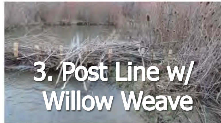
Figure 11. A post line with wicker weave is similar to a starter dam, but acts more like a weir in that water is allowed to flow through the willow branches such that low flows are not over topping the structure and the woven branches may not extend to the top of the posts. These may naturally seal up by trapping sediment and organic material moving downstream or they may be utilized by beaver. Note that beaver have started to colonize this FLWW, as evidenced by the chewed stems on the right of the photograph, aligned parallel to the flow.
